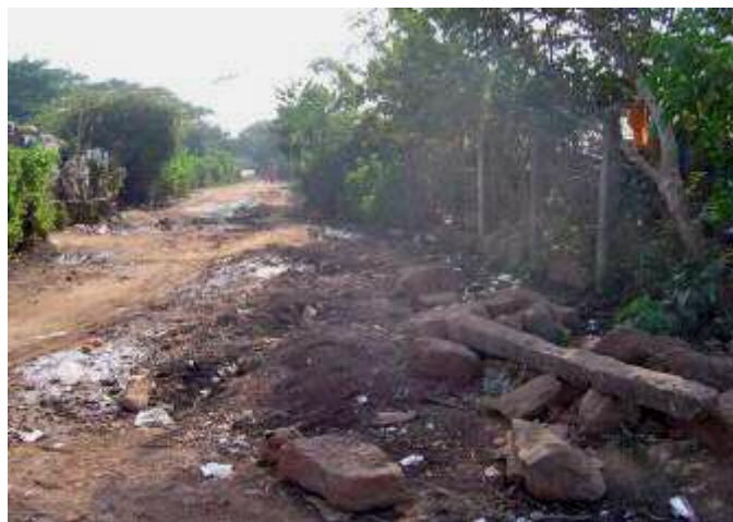
Absence of sanitation and paved road surface
