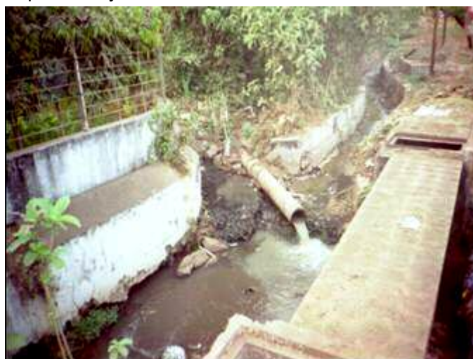
Discharge of raw sewage to open drains
