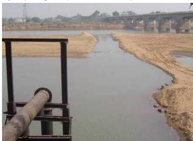
Intake pipes on Kuakhai River - Picture showing channel dug on riverbed to divert main flow
